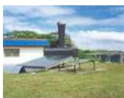
Fig. 4: Photograph of solar dryer system with photovoltaic (PV)
