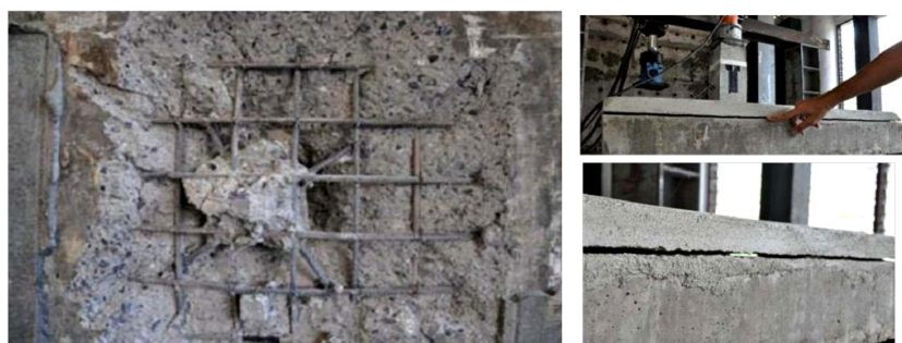
(a) Punching shear failure of slab (bottom view) (b) Delamination of strengthened material for specimen without shear connector
