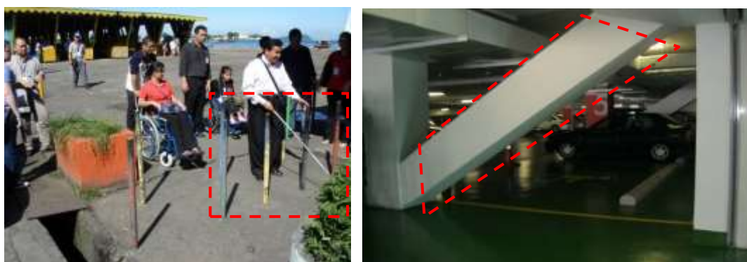
Figure 3: Protruding objects that are hazardous for visual impaired people
