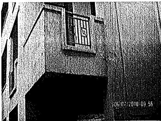
Figure 1. Poor plastering finishes of wall and column (Conventional Method)
