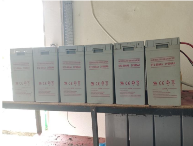
Figure 9. The abandoned battery units from a previous solar project at Kampung Sungai Relang (October, 2023).
