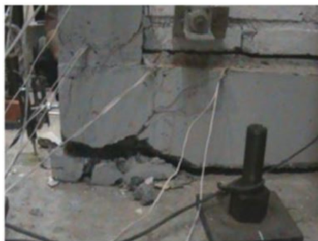
(b) Spalling at the bottom corner of the concrete frame (Triwiyono et al., 2020)
