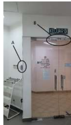
Figure 11. Implementation of smart door at CoEXCyS; a) The circuit box; b) Magnet bar.
