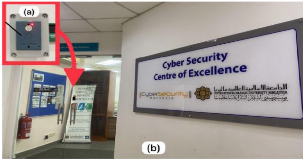
Fig. 13. (a) smart door hardware circuit box. (b) The installation of smart door circuit box at CoExCys office.
