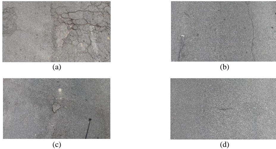
Figure 6. Image samples of road defects captured for each class; (a) crocodile crack, (b) longitudinal crack, (c) pothole, and (d) transverse crack
